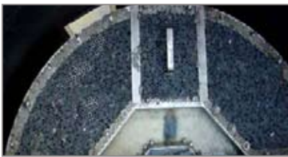
Top of WWETCO Filter before backwash.
