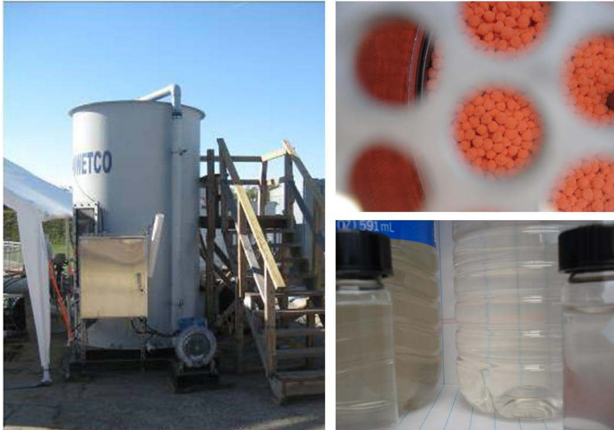
Figure 6. The CMF pilot facilities in Springfield (Ohio) included a filter vessel with media, backwash blower, influent and backwash feed pumps, automatic valves, instrumentation and control panel with PLC. Also pictured are the media bed and representative samples of wet-weather influent and effluent.
